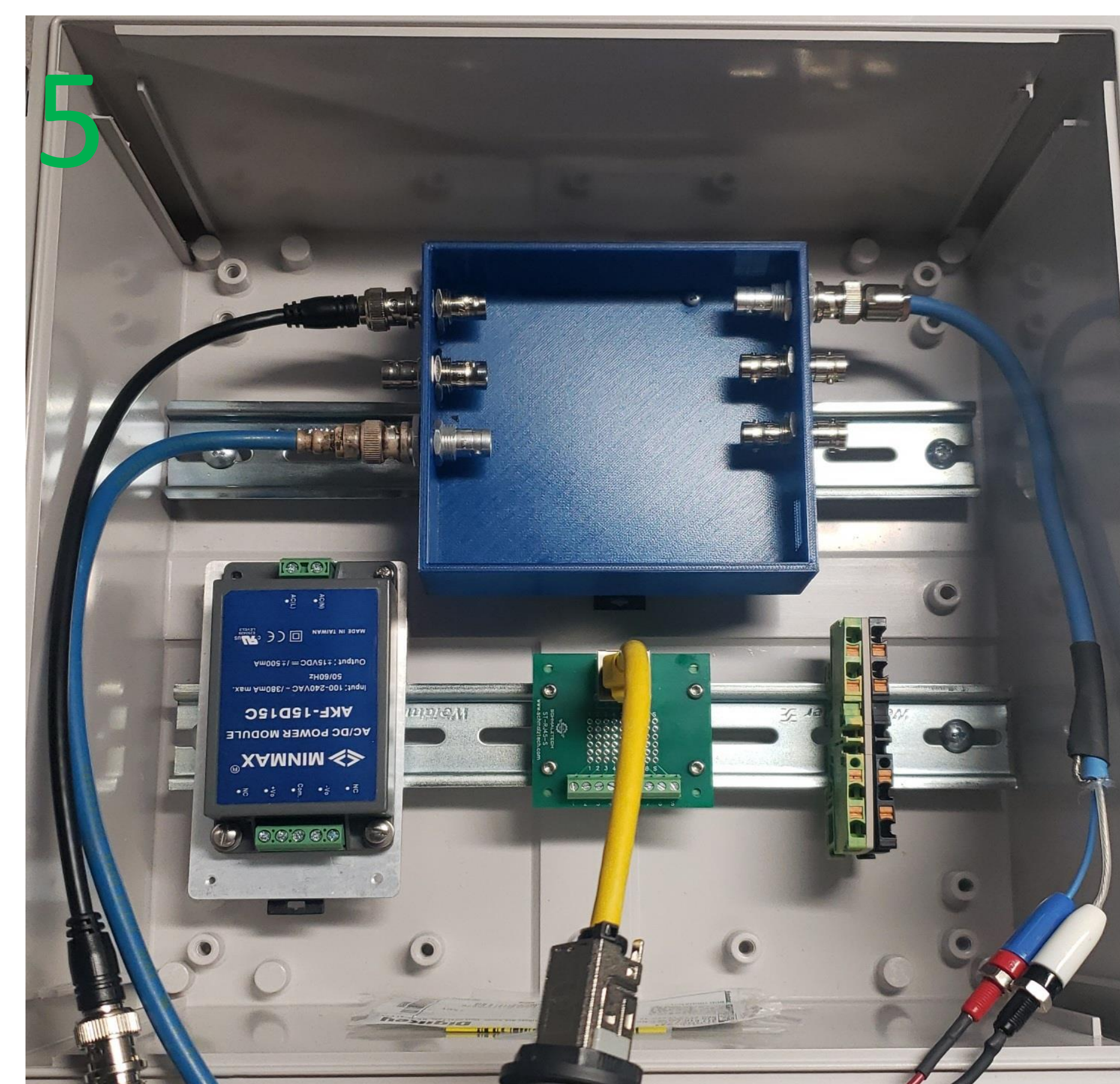
Electronics mounted using 35 mm DIN Rail (Note: Not all wires attached, hole punch outs not yet made at this point)
