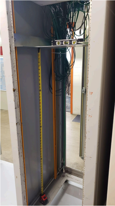
Figure 7. Hardware and equipment used inside the test rack
