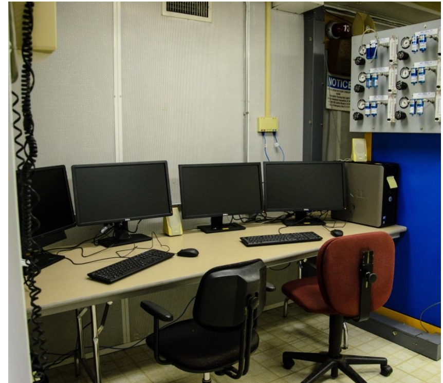
CHL Test Stand Control Room (Climate Controlled, Acoustically Insulated)
