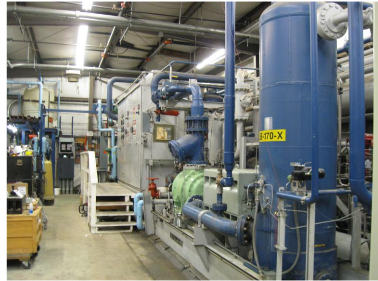
LCW, ICW, Compressor Skid in IB1A
