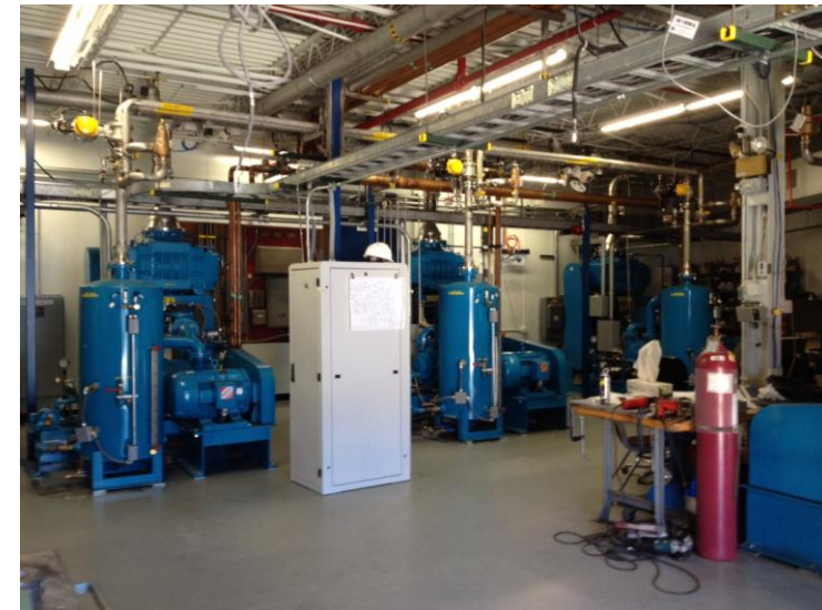
Operational Kinney Pumps in Midway Area
