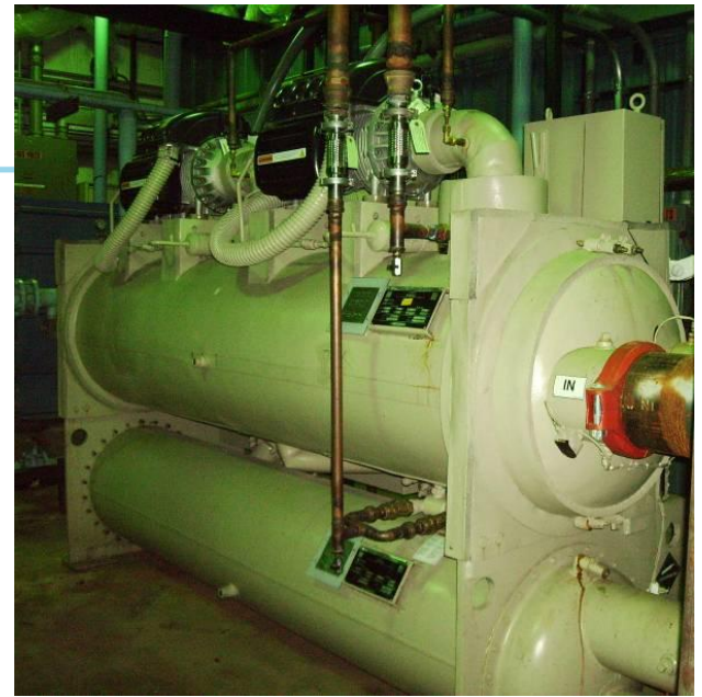
New Chiller in IB1A
