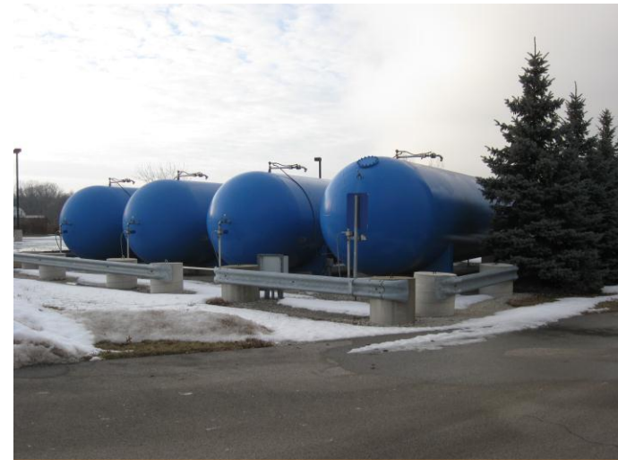
New GHe storage tanks
