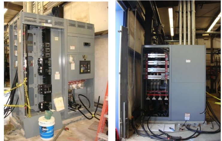
New switchboard and Compressor Soft Motor Starter installed in IB1A, Power Panel installed in Kinney Pump Room
