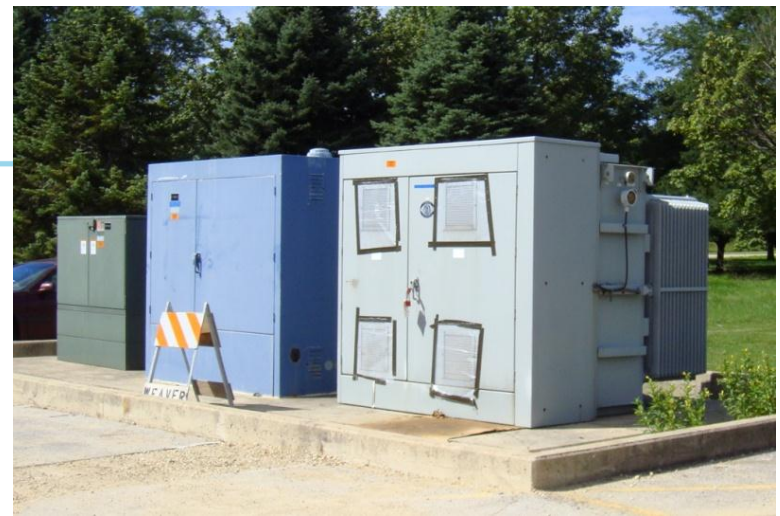
New 1500 KVA transformer installed 2010
