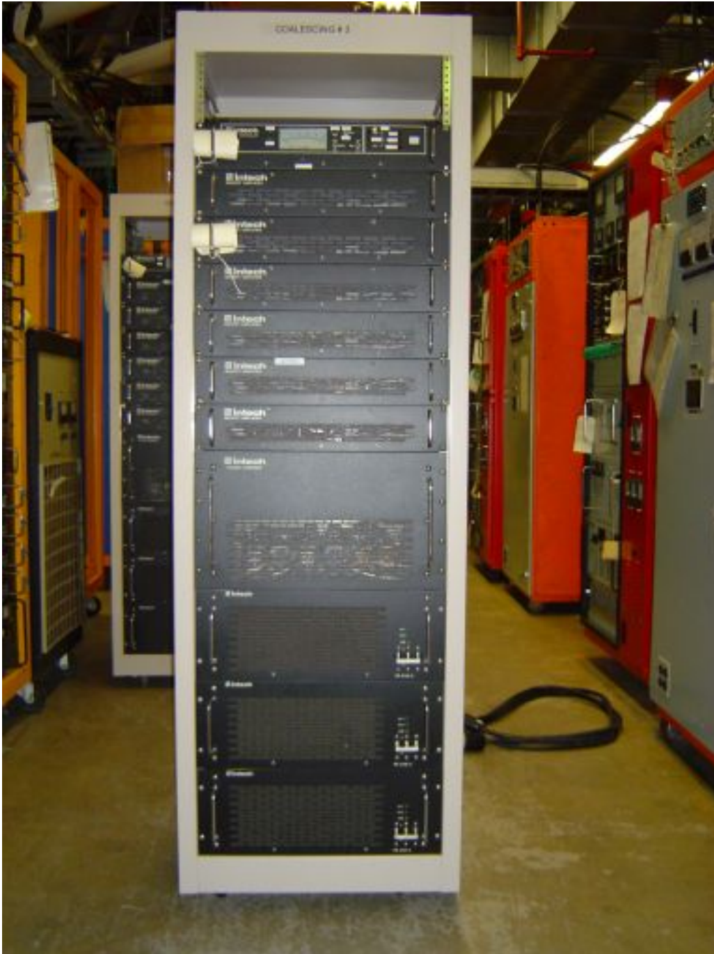
Figure 4.70. Recycler Ring 2.5 MHz Solid State Amplifier. The top rack mount is the controller. The controller also fans out the input from the LLRF to each of the solid state modules. Rack mounts two through seven are 1 kW 2.5 MHz solid-state modules. The fourth from the bottom rack mount is the output combiner for each of the 1 kW solid-state modules. The bottom three rack mounts are the 48 V DC power supplies to the 1 kW solid state modules.
