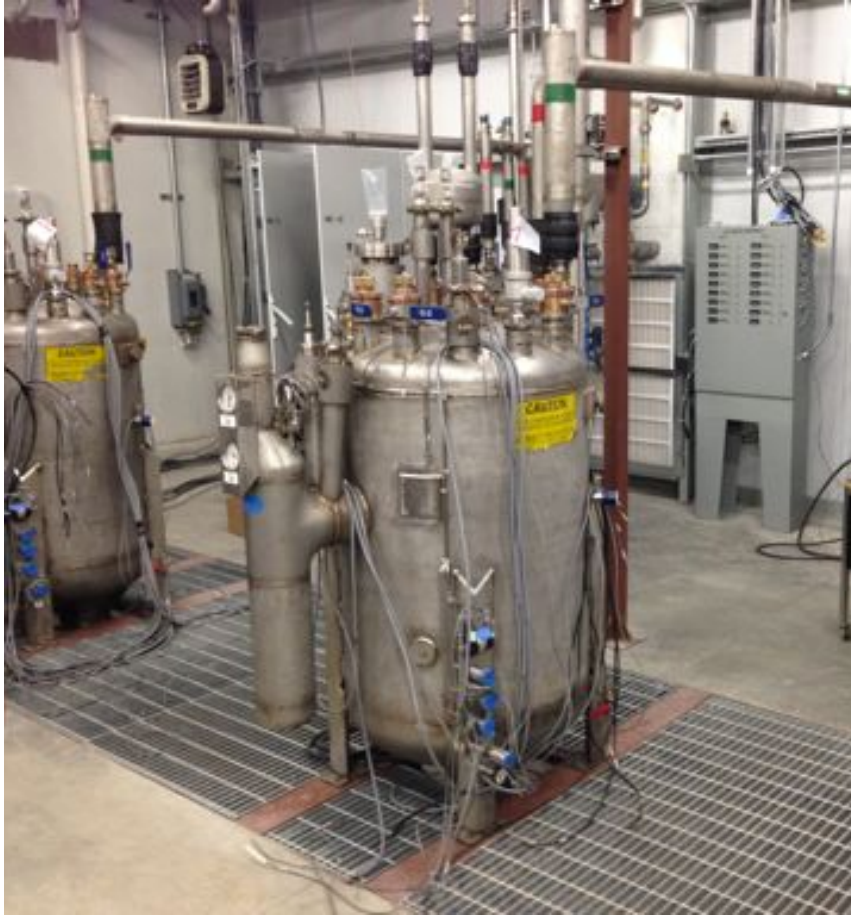
Figure 2.17. Two of the four Tevatron satellite refrigerators that have been installed in the MC-1 building to provide cryogenic helium for the Mu2e and g-2 experiments.
