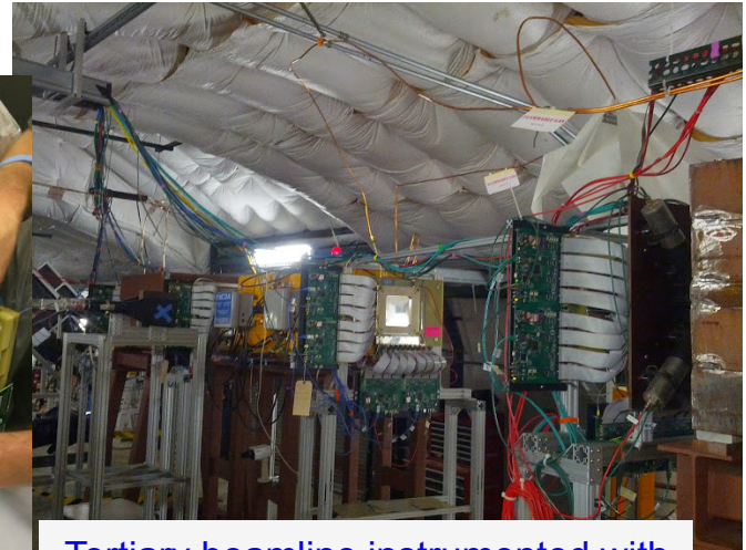
Tertiary beamline instrumented with wire chambers and TOF
