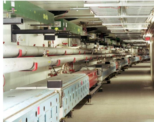
FNAL/Main Injector 120 GeV (1998-present)
